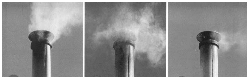
Figure 1: The check your chimney fridge magnet, illustrating (from left to right) excessive, moderate and acceptable smoke levels
